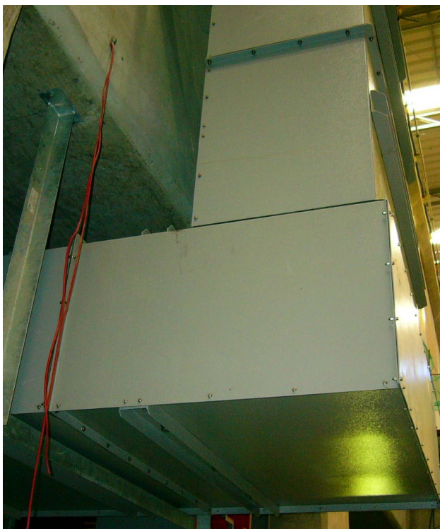
ENGEVIX – UHE CAÇU 13,8kV – 4000A
