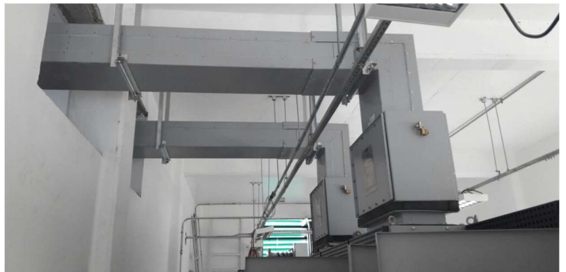
A GUTIERREZ / Amazonas Energia MAUA 3 CCPP B.O.P 480V-3200 A
