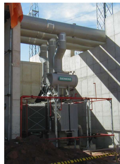
PROMON/N.Odebrecht/A.Gutierrez UTE NORTE FLUMINENSE - 780MW 3x 15kV-10000 A(GT) 1x 23kV-10000 A (ST)
